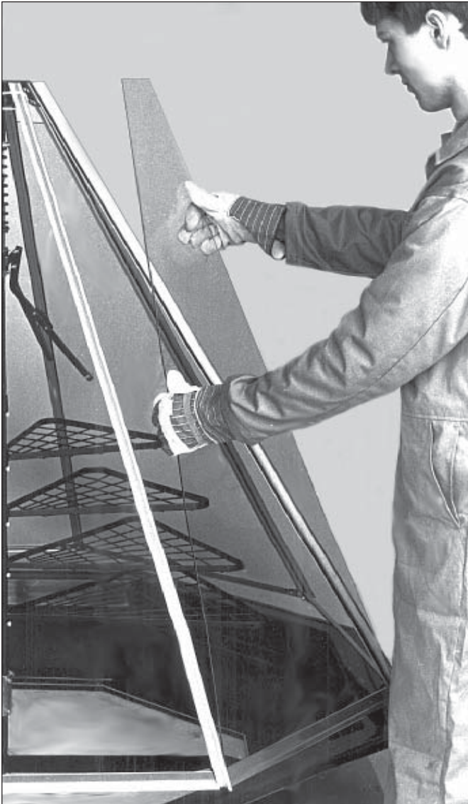
2.13 Fit a glass panel to a frame adjacent to the door frame. (Take care not to glaze the door-frame itself since it is fitted with the removable polycarbonate panel).
